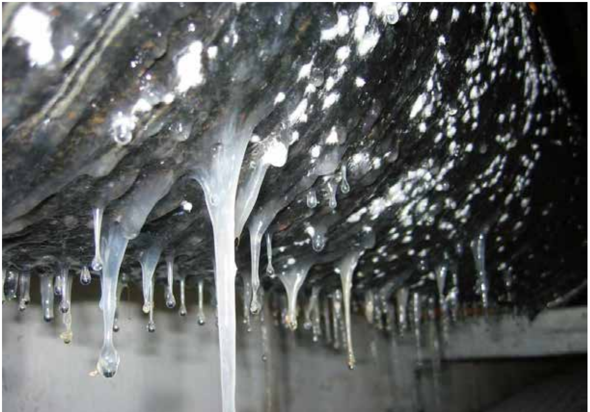
It should not look like this: insulation which works well at first, but on which condensation or – as here – even ice forms after the equipment has been in operation for a while
